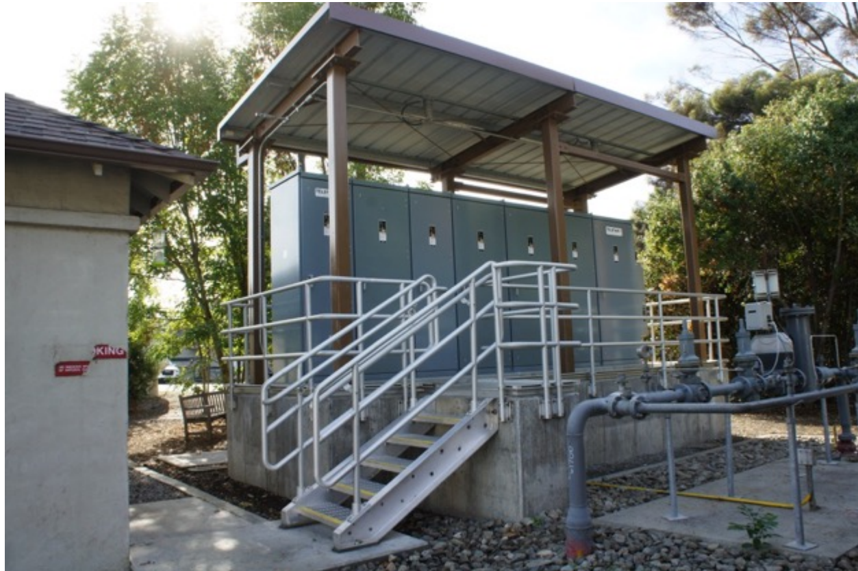
Elevated power distribution equipment at the RWQCP
