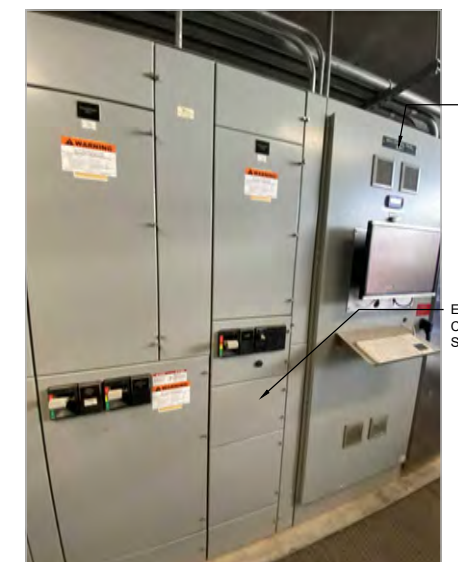
① EXISTING MCC PHOTO
