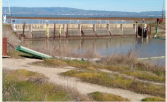
The Palo Alto Flood Basin tide gate structure is one part of the levee system surrounding the City's Flood Control Basin. It is planned for replacement by 2026.
