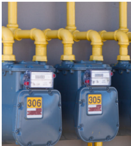
The City of Palo Alto natural gas distribution system is sensitive to flood hazards.
