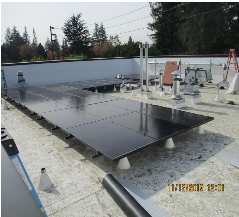
Roof-top mounting of photo voltaic panels on horizontal supports.
