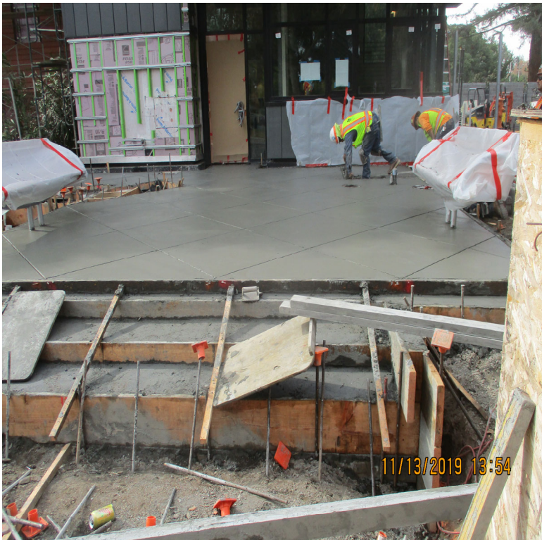
Entry plaza concrete placement at Newell Road entrance to the fire station.
