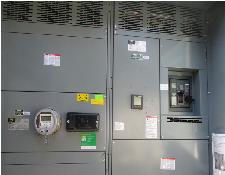
Newly Installed Switchgear and Meter
