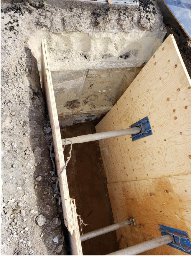
Trenching for duct bank along Ash St. including tie-in at existing vault.
