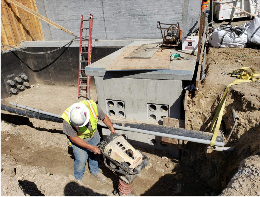
Electrical vault installed onsite.
