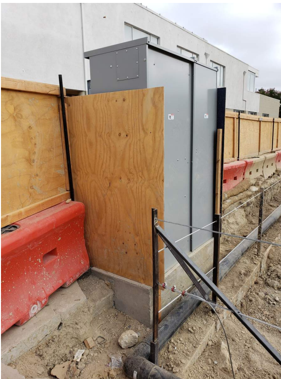
Temporary construction power switchgear installed.
