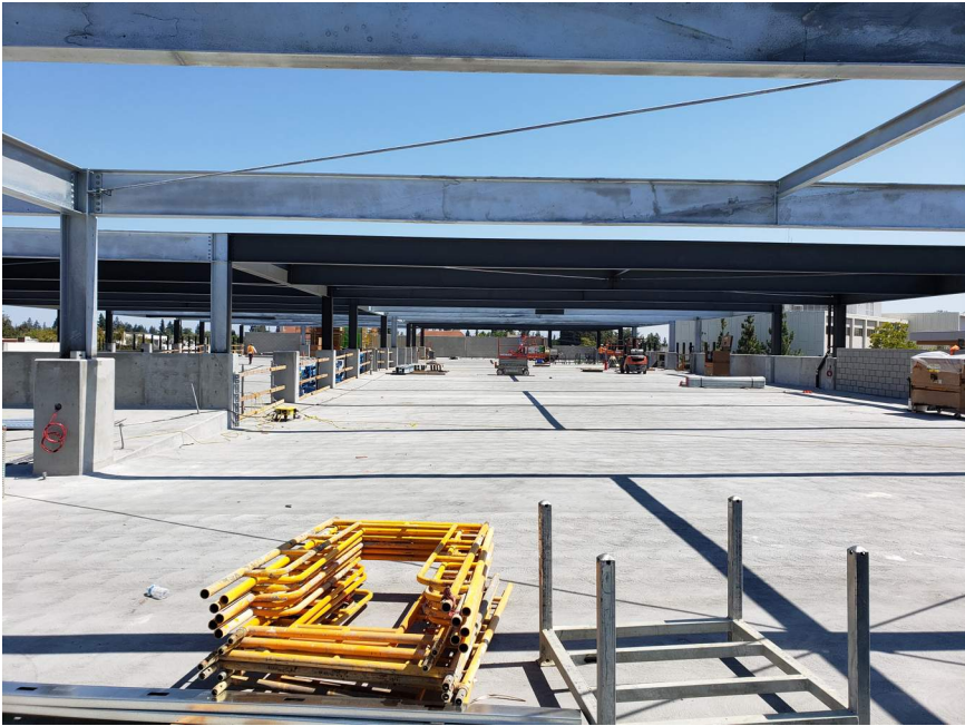
Painting of structural steel for future PV system on roof level ongoing.
