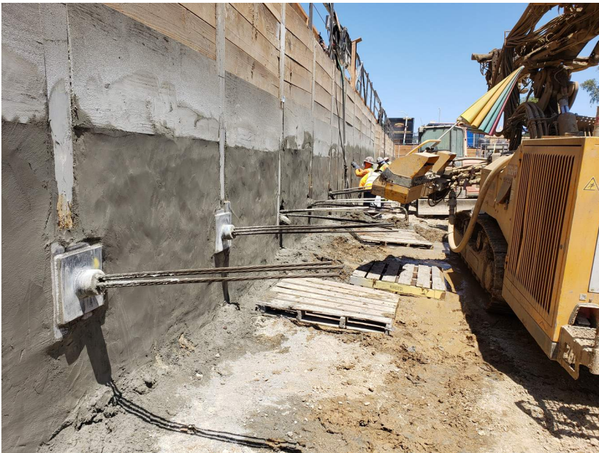
Tieback testing and stucco being applied to shoring wall (to provide smooth substrate for application of waterproofing membrane).
