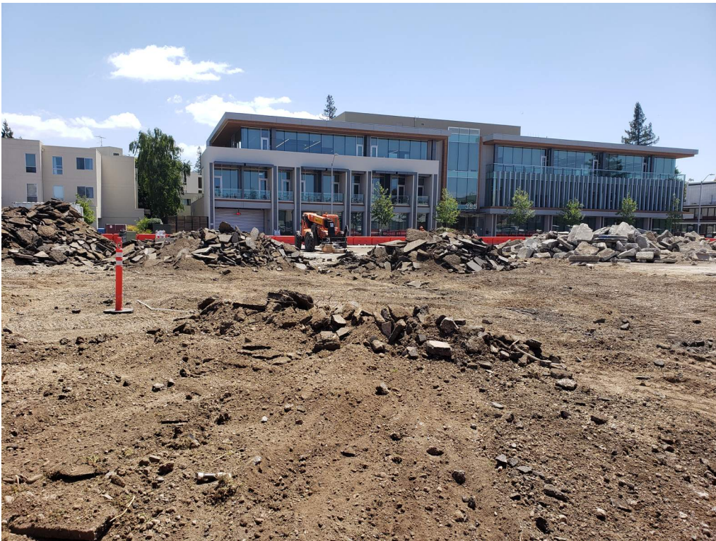
AC and Concrete have been demolished and off hauled at lot C-7.
