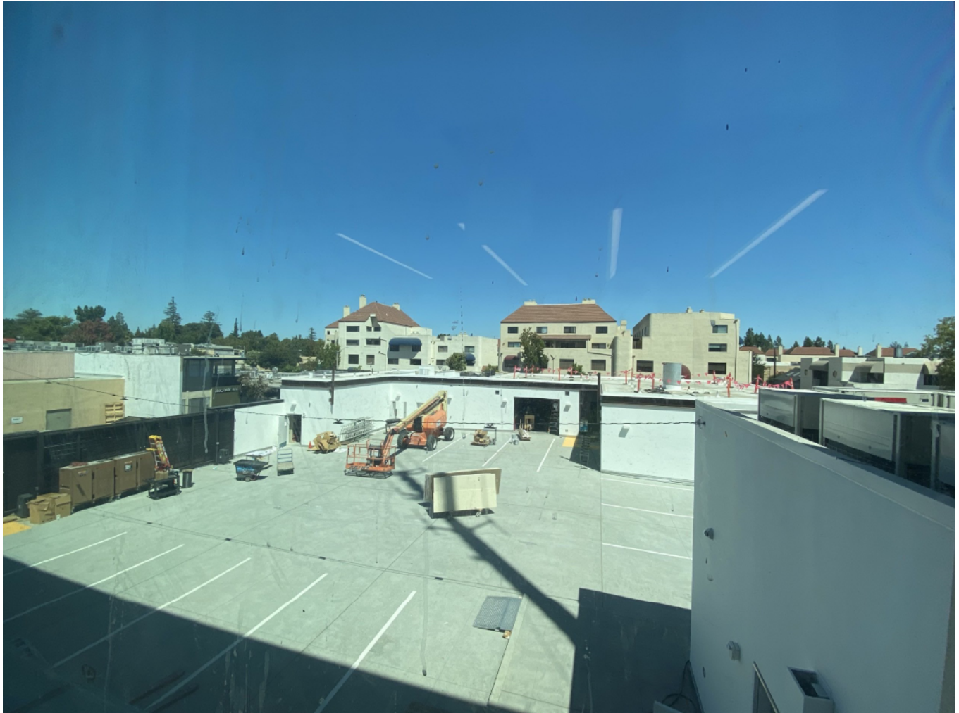
L2 View of Utility Yard.
