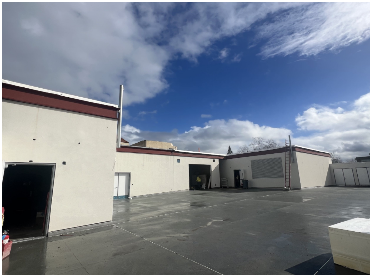
View of utility yard.
