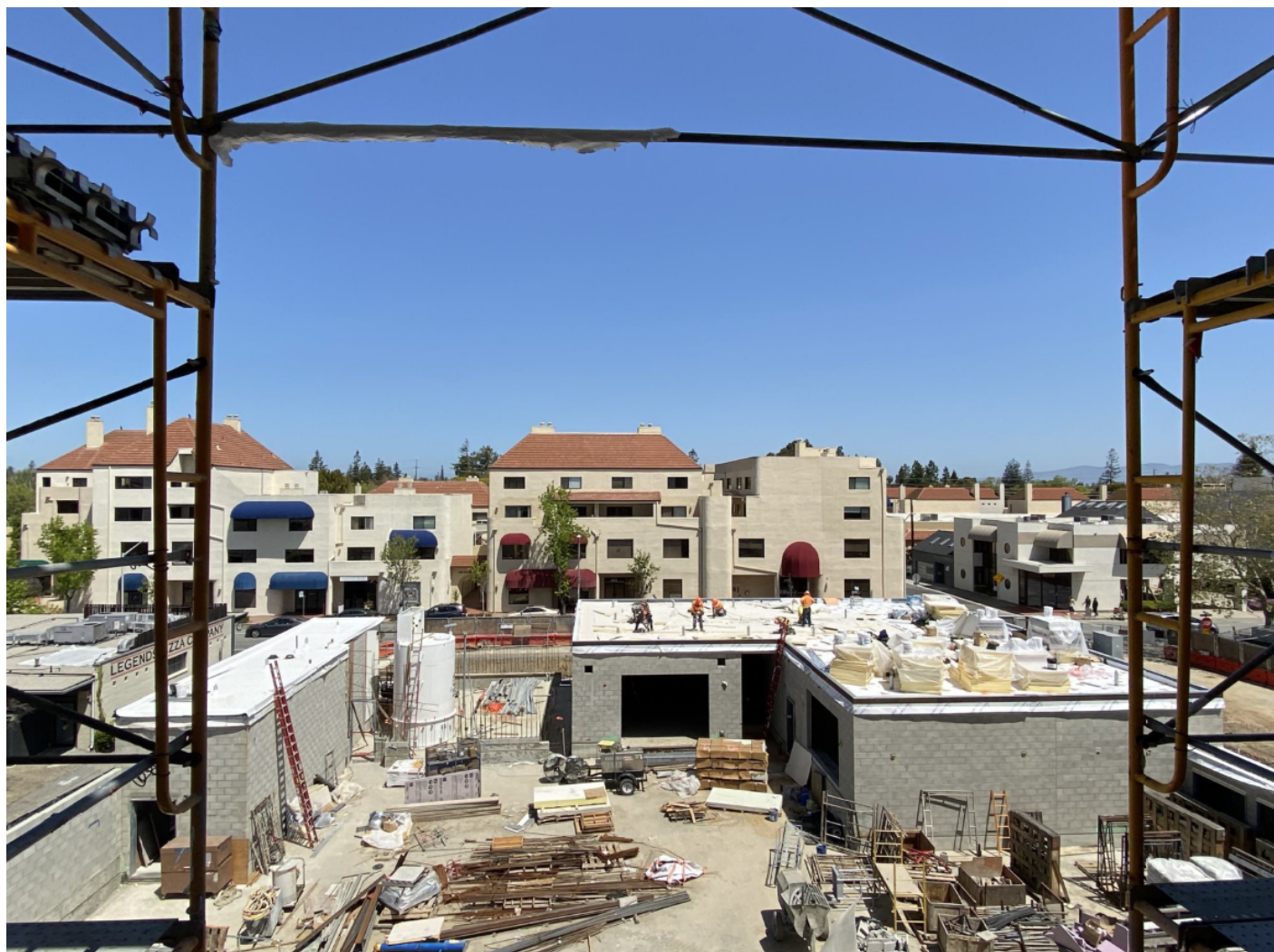
Utility Yard Installation view from 3 rd Floor.
