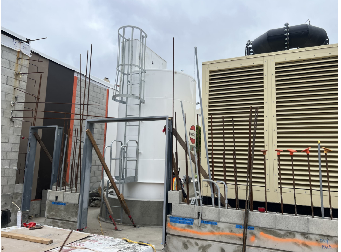
View of view of Fuel Tank and Generator Installation in the Utility Yard.
