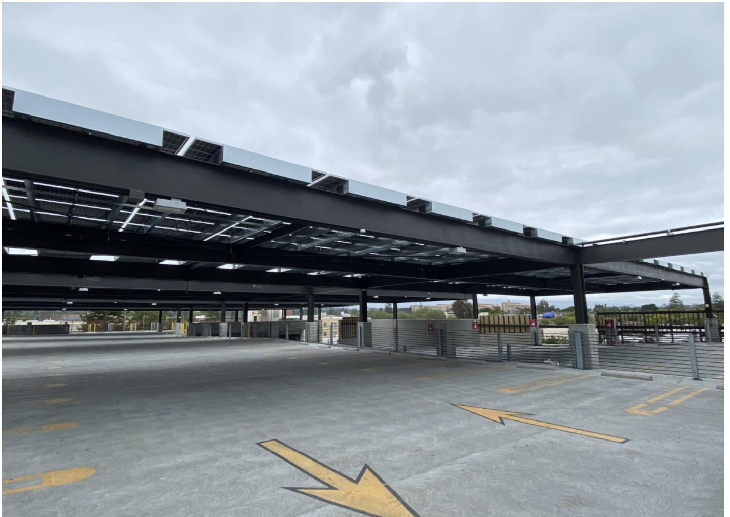
View of PV Installation Fourth Floor.
