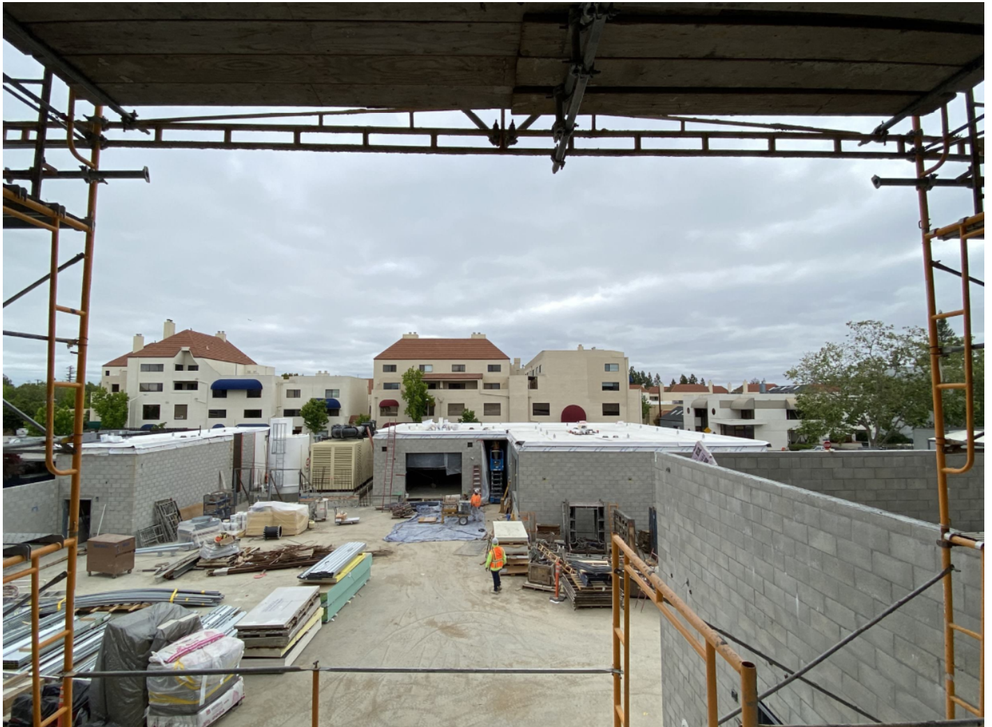
View of Utility Yard from Level 2.
