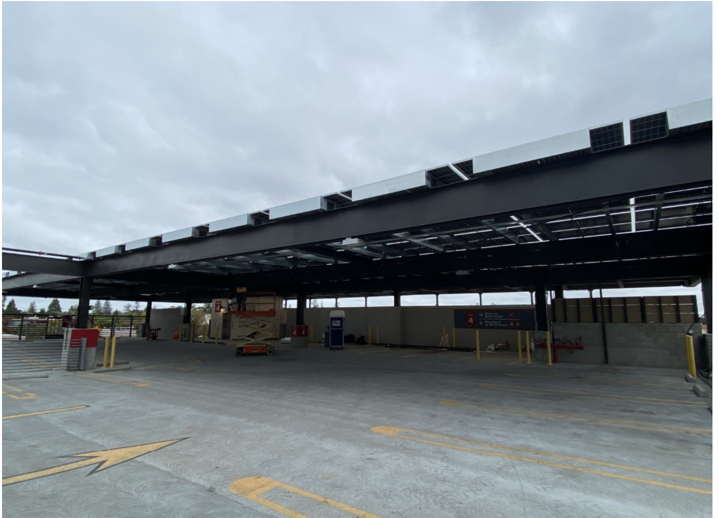
View of PV Installation Fourth Floor.
