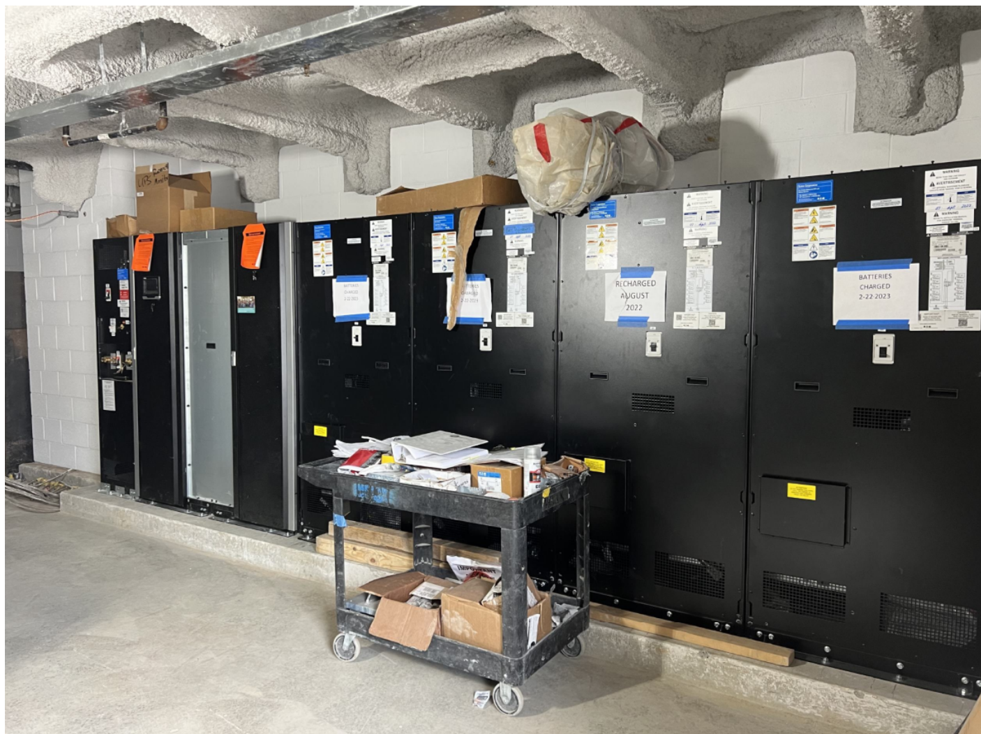
View of Equipment in Emergency Electrical Room.
