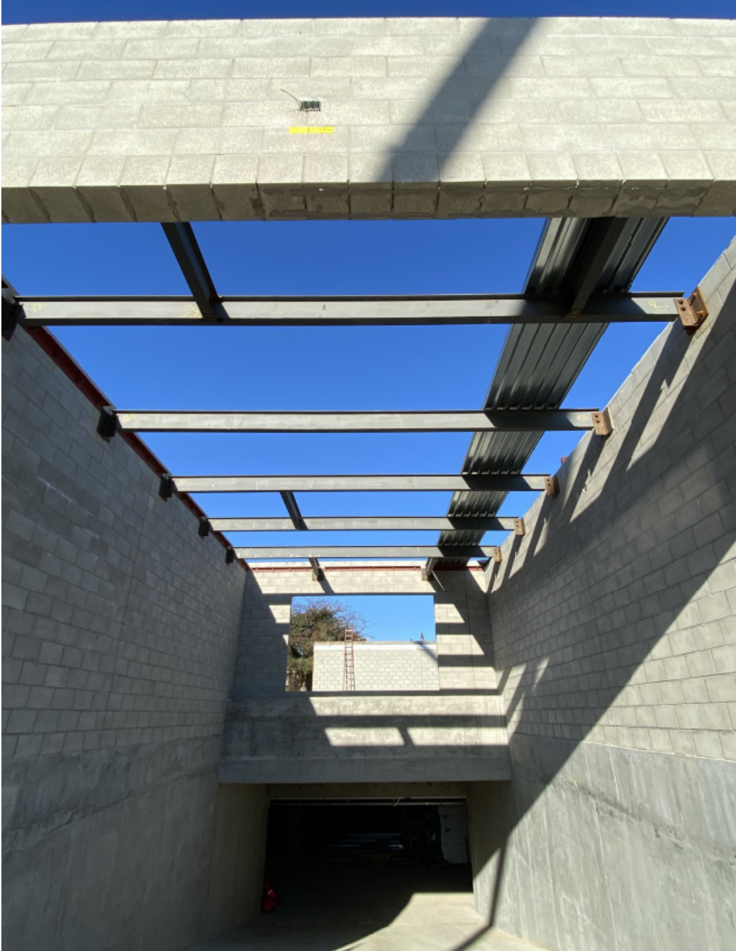
View of driveway ramp of steel installation and metal decking being prepped for layout.
