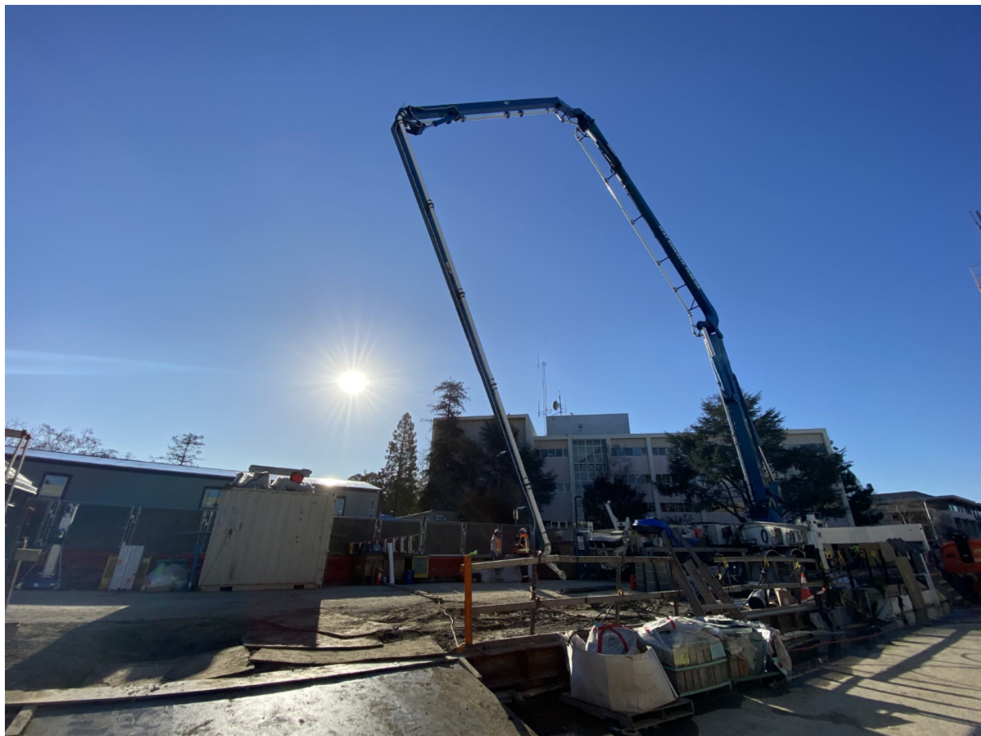
View looking towards Sherman Ave within project site of Concrete pump being prepped for concrete pour of L2 Electrical Room and Entry topping slab.
