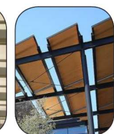
M7 PV Panel Sup- ported by Paint- ed AESS framing
