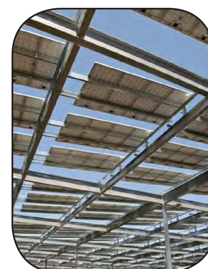
M18 PV Panel Supported by Painted AESS framing
