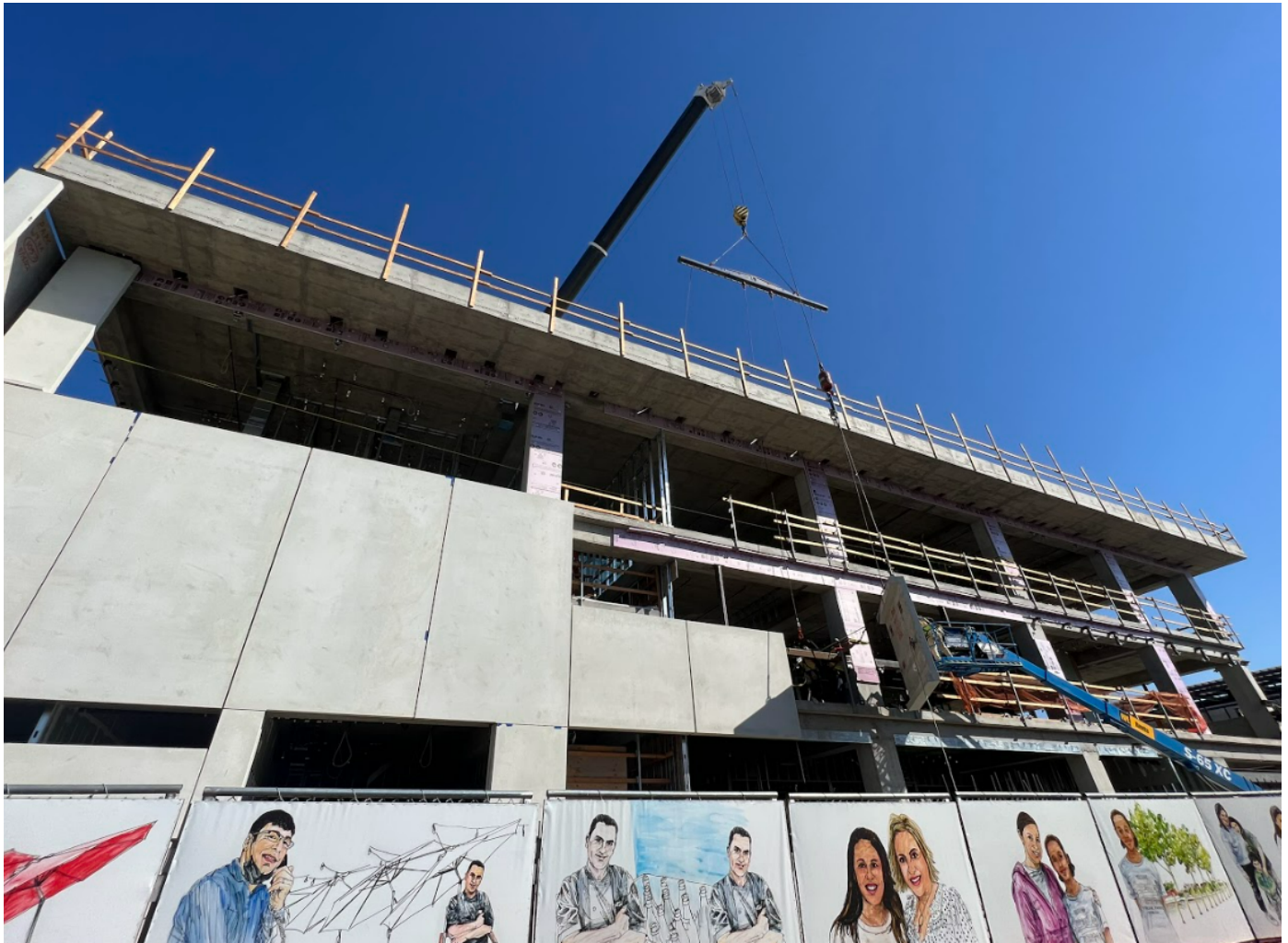
Closeup view of Precast Panels being installed on the North elevation. View from Jacaranda St.
