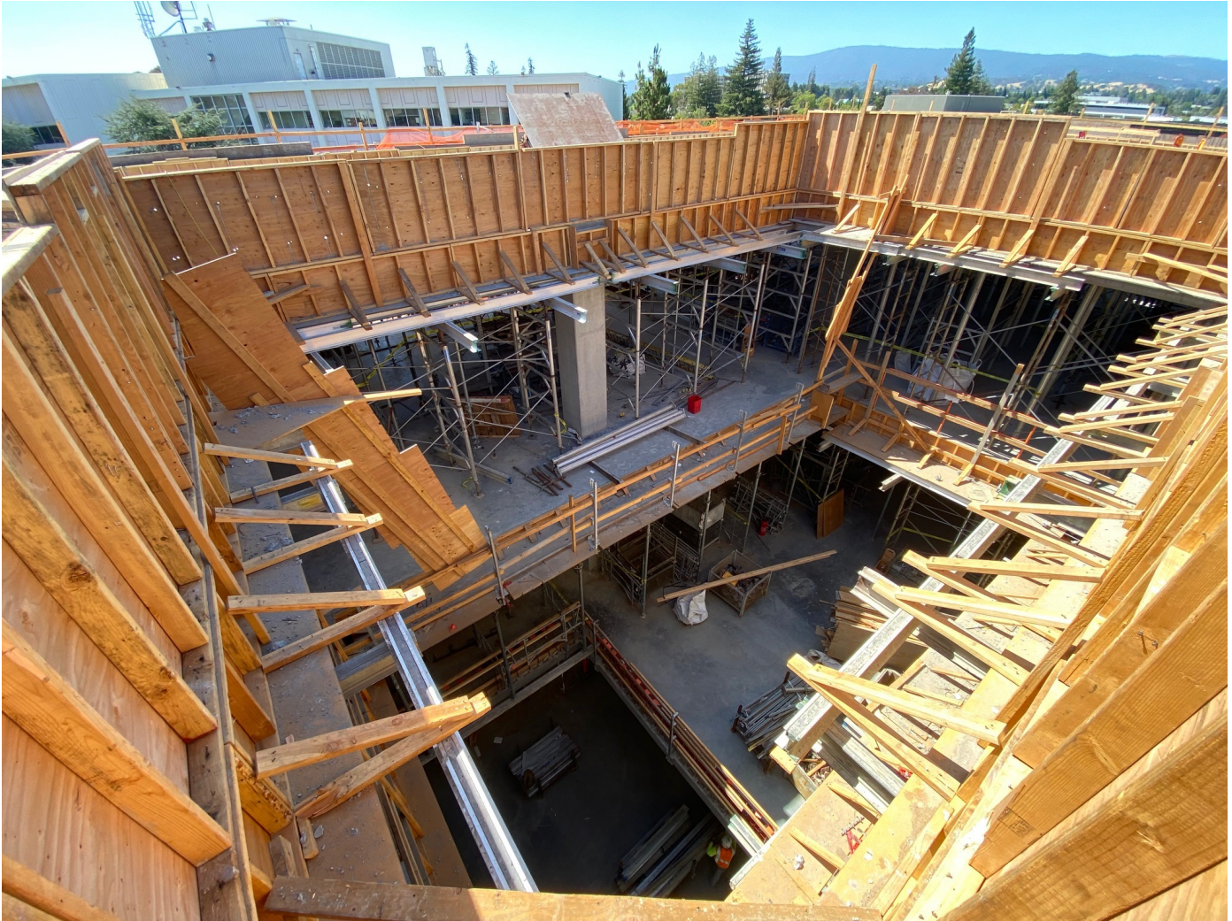
Concrete formwork in place on Level 4 (roof) and looking down through future skylight.
