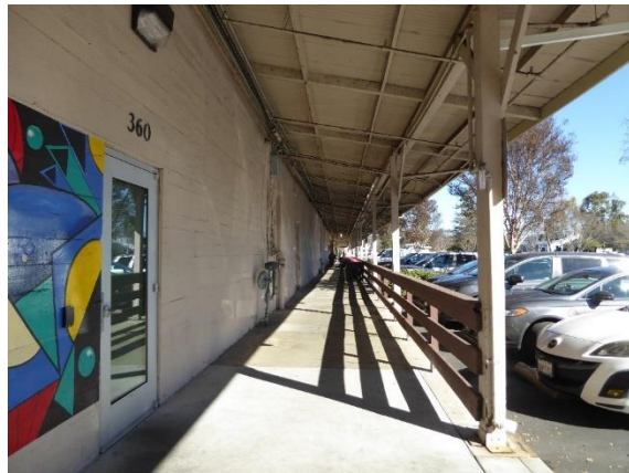
Figure 8. A shed awning with wood post-and-beam supports extends nearly the full length of the southeast façade. View northeast.
