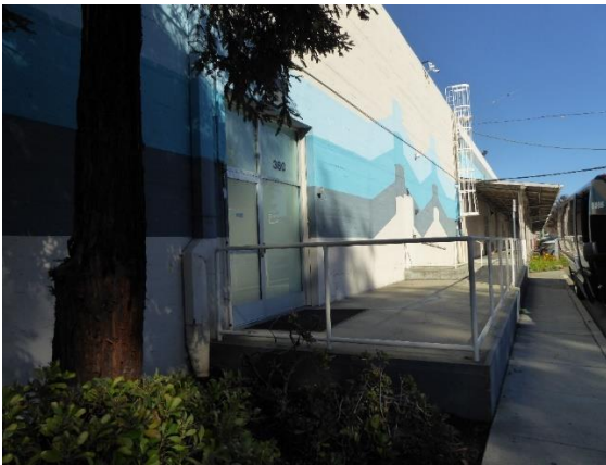
Figure 7. Concrete platform extends from an aluminum frame glass entry at the far south end of the southeast façade. View northeast.
