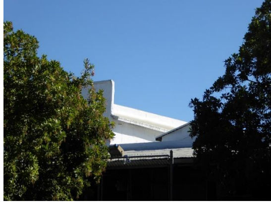
Figure 24. Rooftop parapet and small gabled roof in middle section of northwest façade. View northeast.
