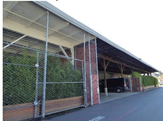
Figure 32. Wood post-and-beam construction under the awning at the south end of the northeast façade. View south.
