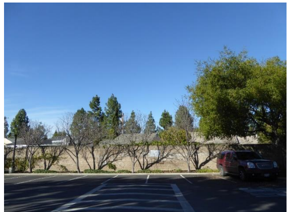
Figure 50. A concrete block wall borders the parcel to the northwest. View northwest.
