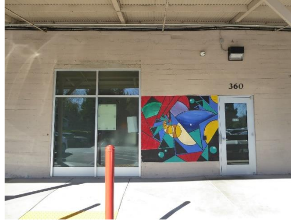
Figure 12. Many historic doors and openings have been replaced with aluminum frame glass windows and doors. View northwest
