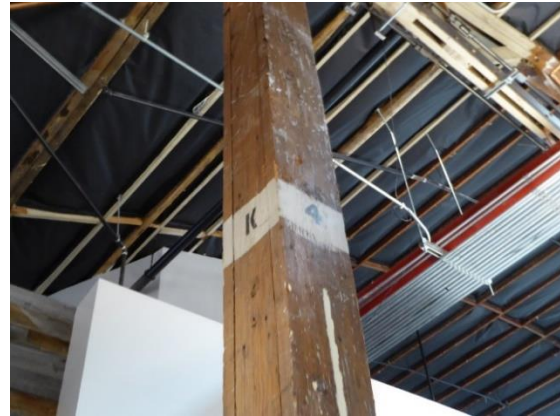
Figure 44. Painted numbers and letters remain visible on unfinished wood posts in 380 Portage Avenue.
