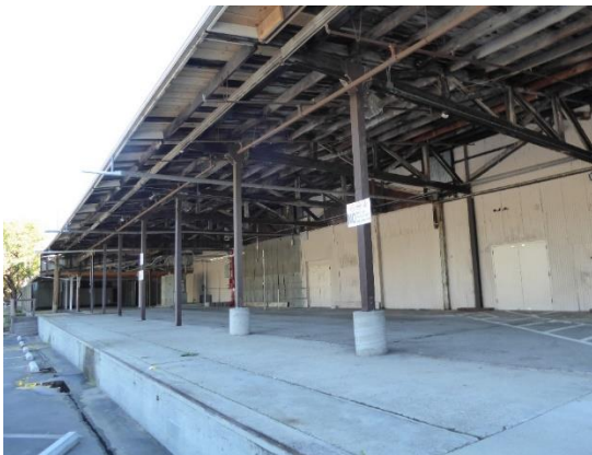
Figure 27. A portion of the concrete loading platform or cooling porch with its shed awning and wood post-and-beam supports in the middle section of the northwest façade. View northeast.
