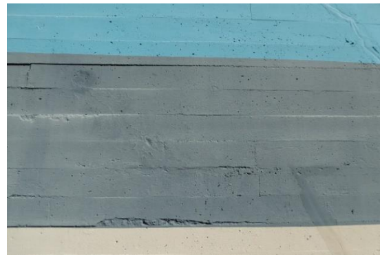
Figure 34. Painted board formed concrete on the southwest façade. View northeast
