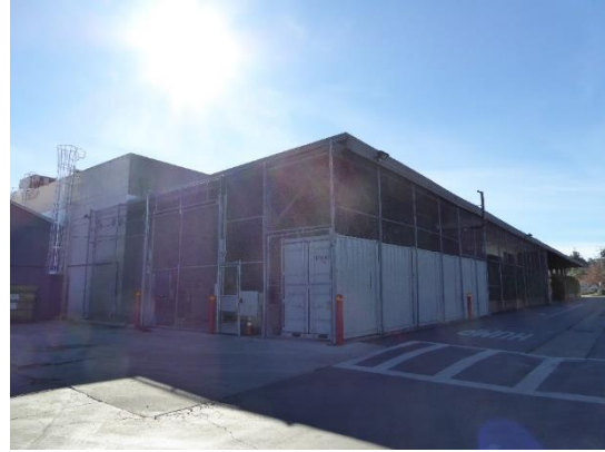
Figure 30. Double-height concrete structure with a wide flat-roofed awning and chain-link fence at the far south end of the northeast façade. View south.
