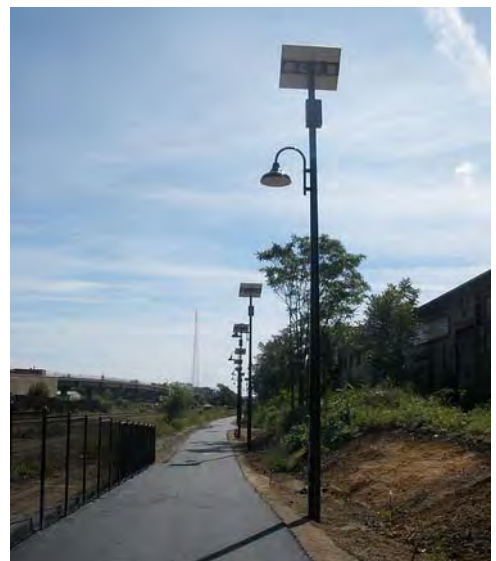
Exhibit 1 Solar lighting is used along the Metropolitan Branch Trail in Washington, D.C. Source: http://www.thewashcycle.com
