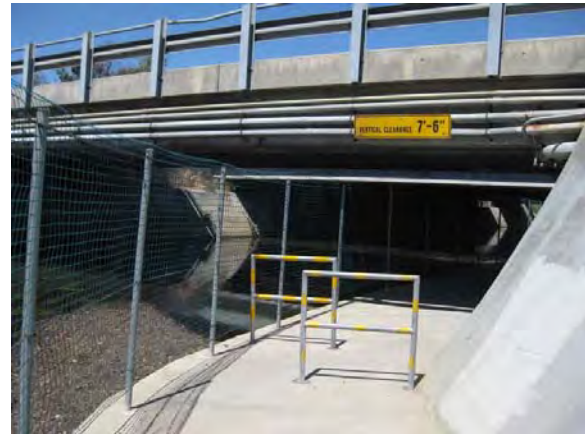
Despite being open only five months out of the year due to seasonal flooding, the Adobe Creek Underpass carries an estimated 43,000 annual users.
