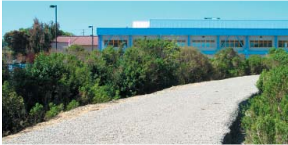
Crushed stone trail along the levee near San Francisquito Creek. Note how stone is contained by plastic edging. Because the trail is above the earth level, the plastic edge is uneven.
