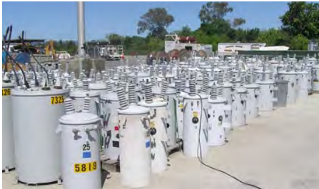
These Utility Department transformers are stored at the MSC—on a huge concrete pad designed and built specifically for that purpose
