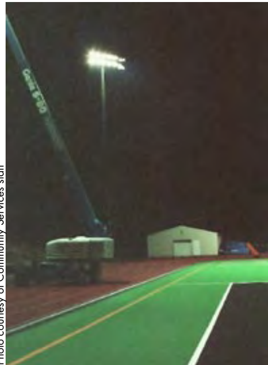
The new light field and security lights represent significant improvements in terms of energy efficiency, efficacy of field illumination, and reduction in glare and off site spill factors.
