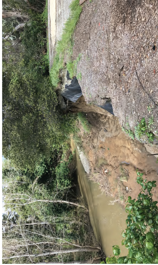
View 3. Northwestern view of the creek bank failure and San Francisco Creek, on top of the creek bank.
