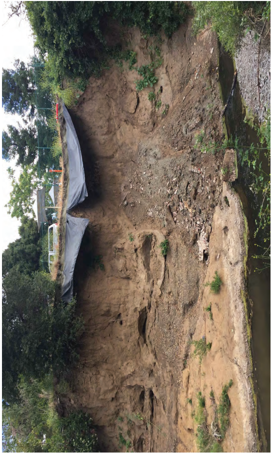
View 1. View of the creek bank failure at the project site, looking across San Francisco Creek.
