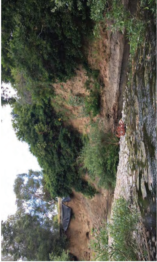
View 2. View of the creek bank failure and San Francisco Creek, looking north from within the creek bed.
