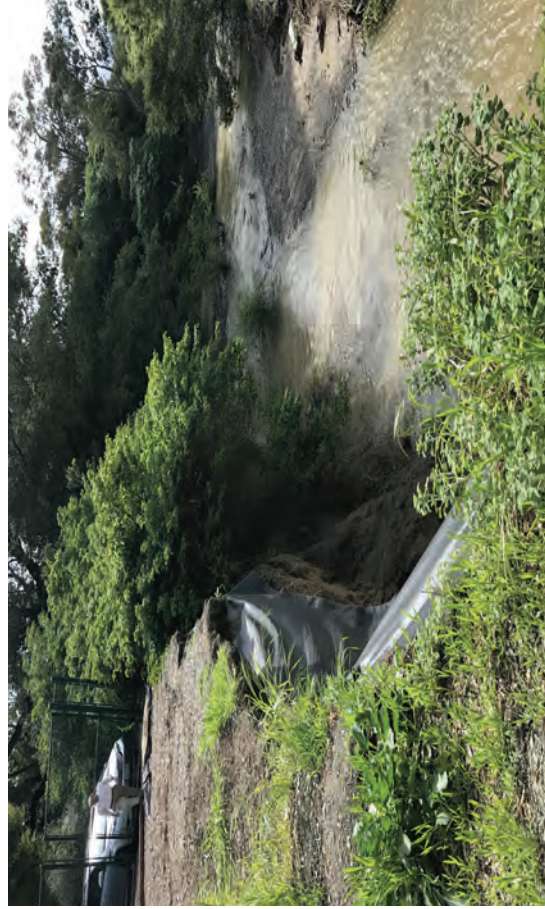
View 4. Southeastern view of the creek bank failure and San Francisco Creek, on top of the creek bank.
