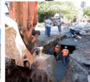
New storm drain pipes were installed along Channing Avenue in 2011 to reduce frequent street flooding along this important vehicle and bike corridor.
