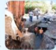
New storm drain pipes along Charming Avenue reduce street flooding along this important vehicle and bike corridor.
