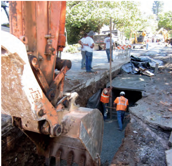
New storm drain pipes were installed along Channing Avenue in 2011 to reduce frequent street flooding along this important vehicle and bike corridor.
