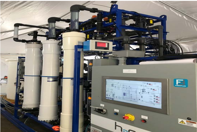
Filtration system testing unit
