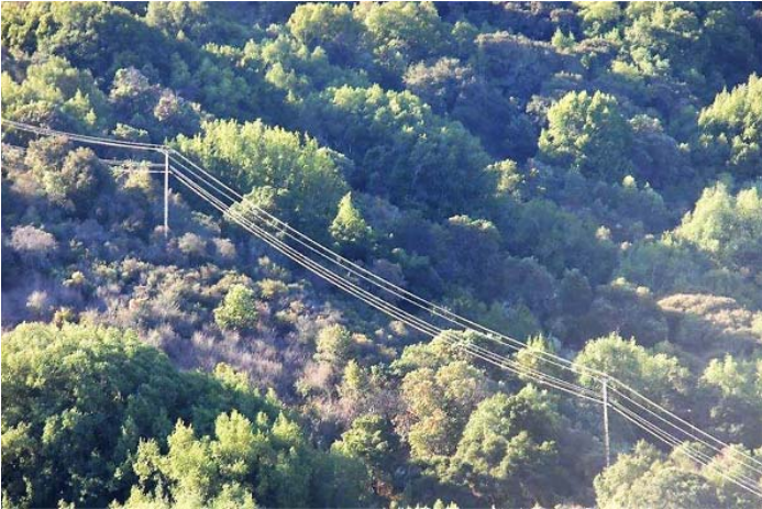
Overhead electric lines in Foothills Park
