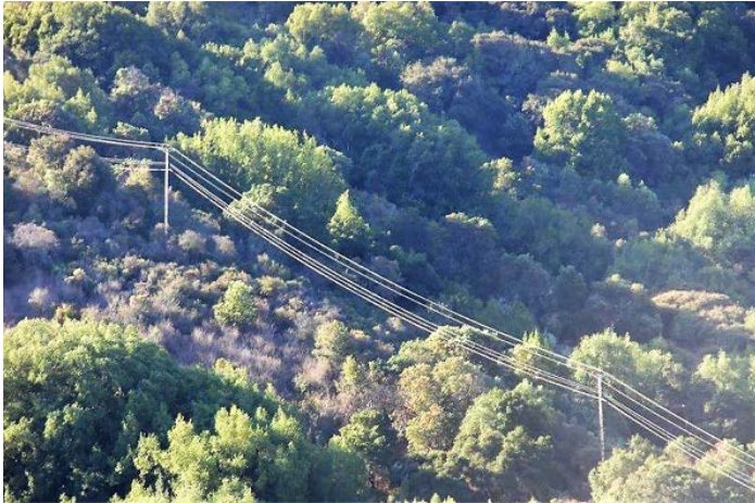
Overhead electric lines in Foothills Park
