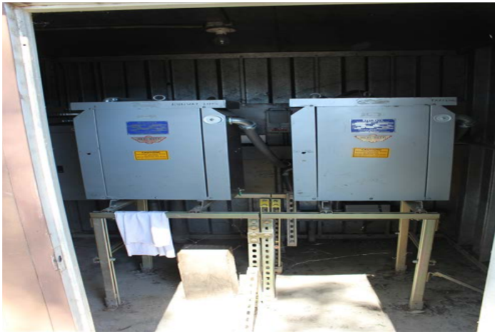
Airfield Electrical, July 2017
