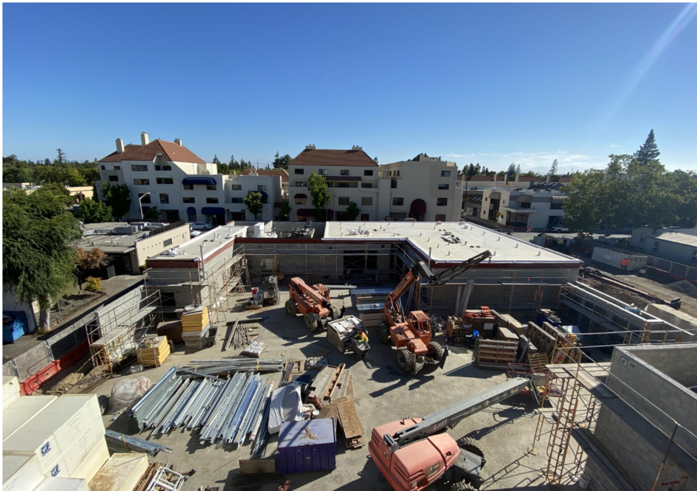
View of Utility Yard from Third Floor.
