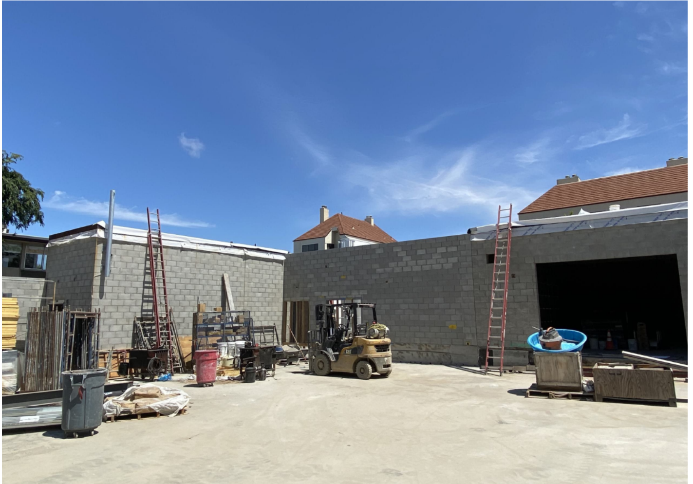
View of Utility Yard.
