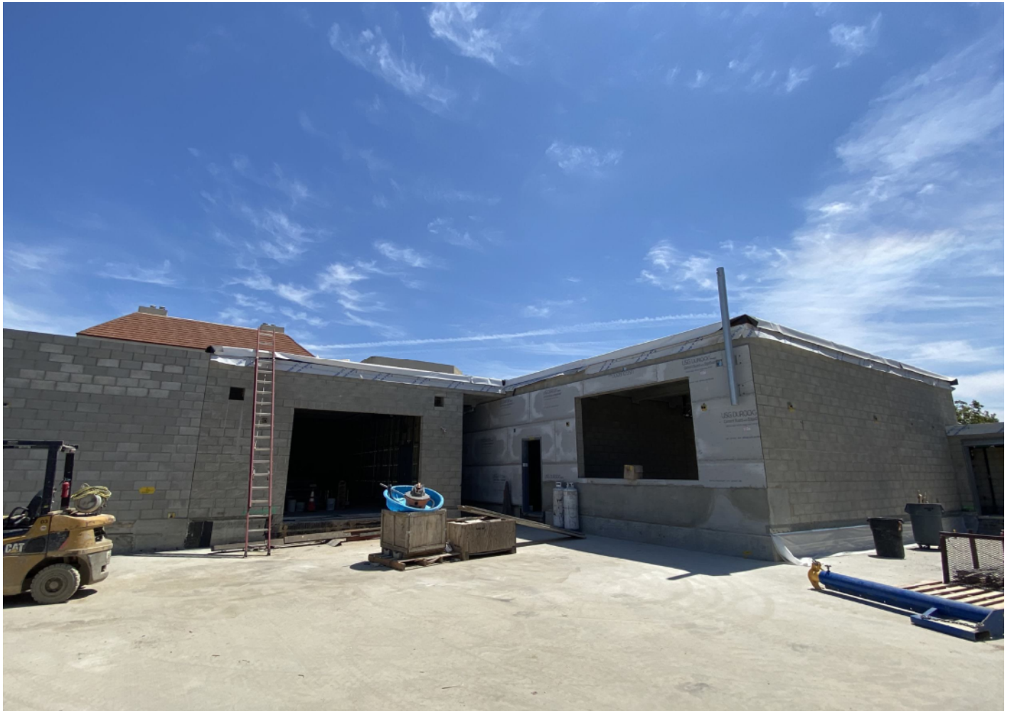
View of Utility Yard.
