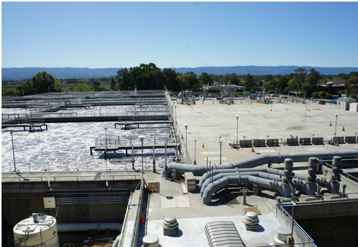
Looking West from Fixed Film Reactors
