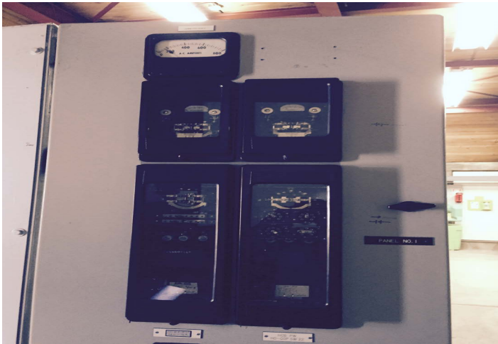
Aging electric equipment
