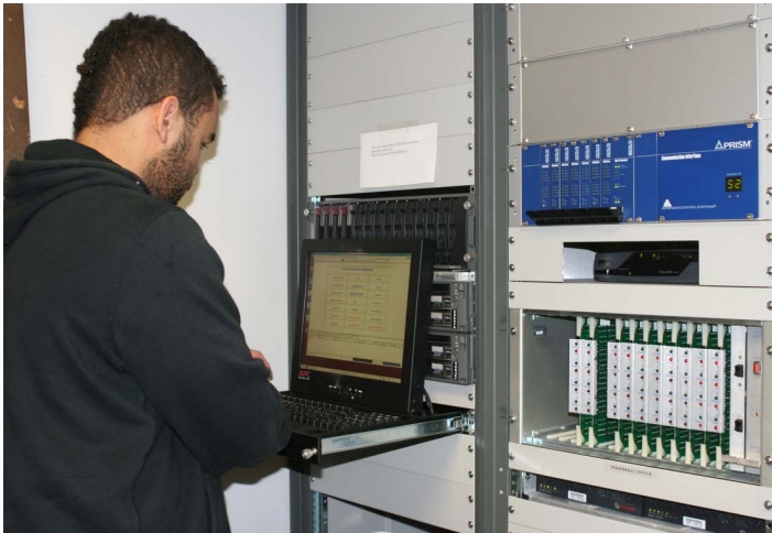
SCADA Technologist configuring SCADA software
