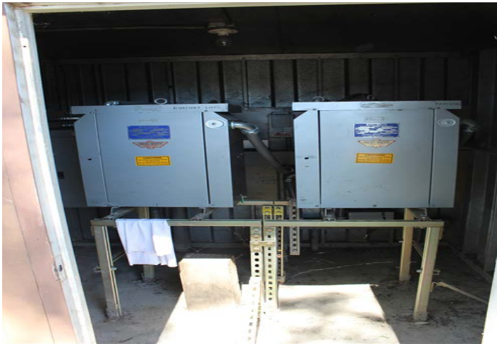
Airfield Electrical, July 2017
