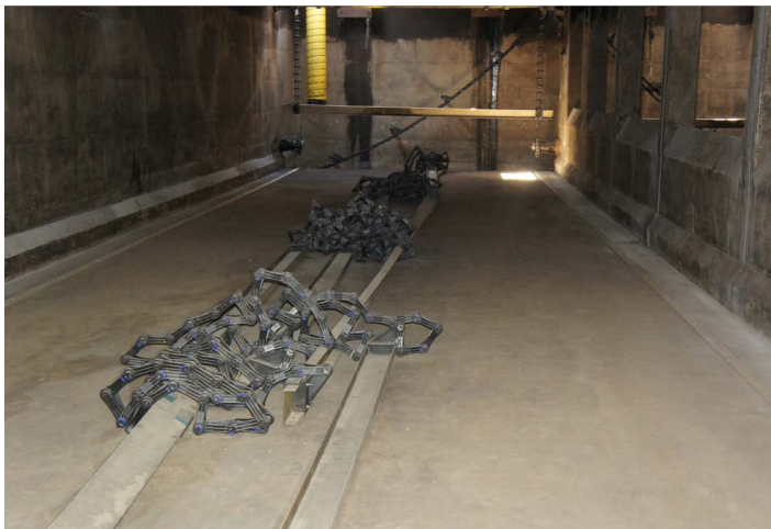
Primary Sedimentation Tank
