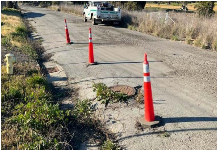
Deteriorating Condition of Airport Access Road
