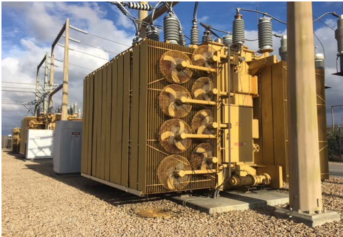
Colorado Power Substation
