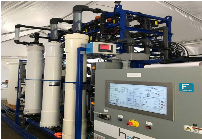
Filtration system testing unit
