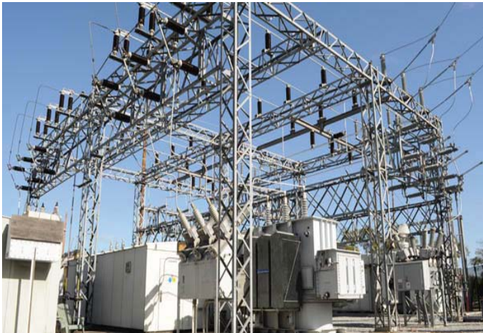
Electric Substation transformer and bus structure
