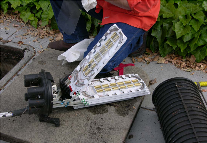
Fiber optic splice closer ready for inspection and work
