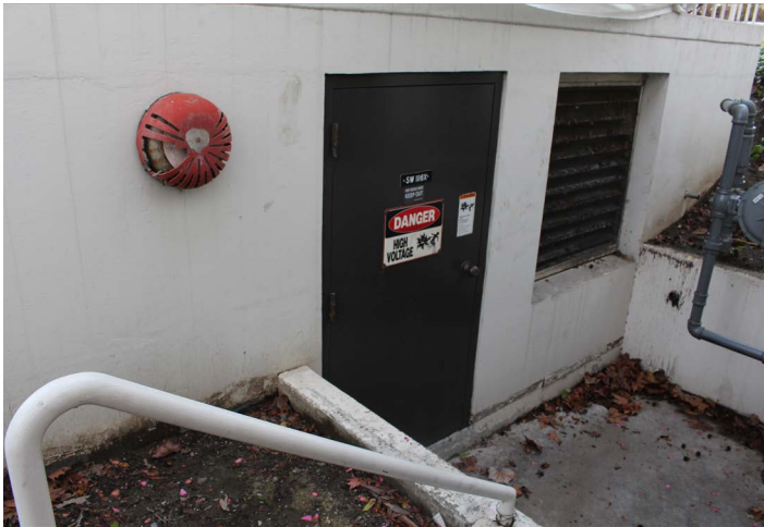
Electrical System Access Door at City Hall
