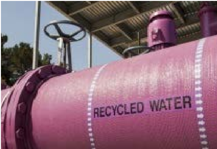
Recycled water piping
