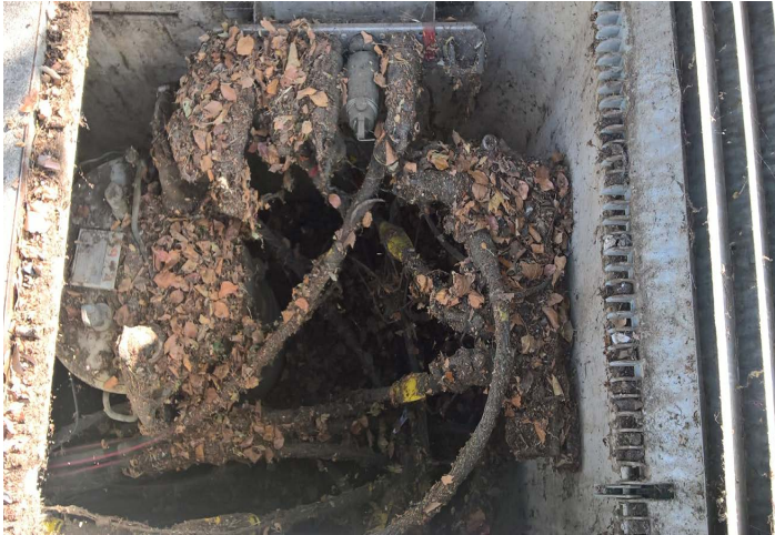
Underground Utilities Enclosure
