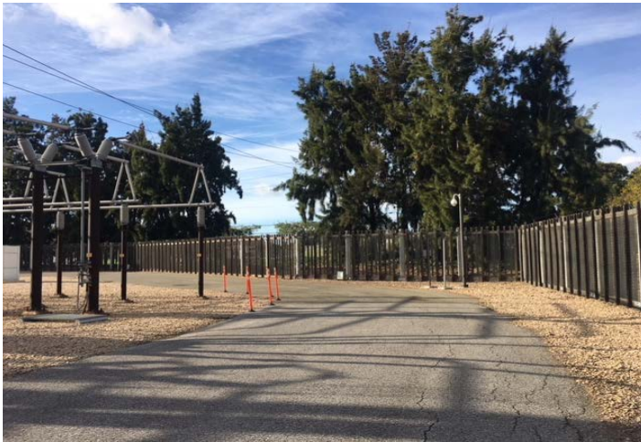
Colorado Electric Substation Driveway
