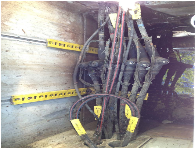
Electric underground cable vault
