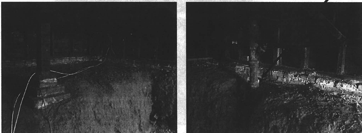
Figures 24 and 25. Views of the foundation from inside the half-basement. Brick piers and timber posts are visible in the left image. The right image shows loose bricks and efflorescence at the crib wall, particularly where the sanitary utility line meets the foundation ( Photo: PAST Consultants ).
