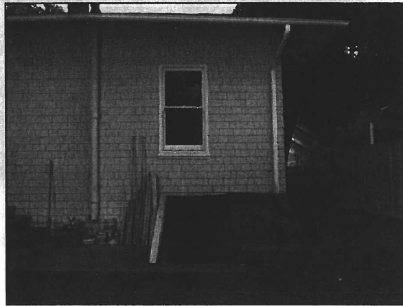
Figure 28. Downspouts discharge water against the building, shown by an arrow ( Photo: PAST Consultants ).
