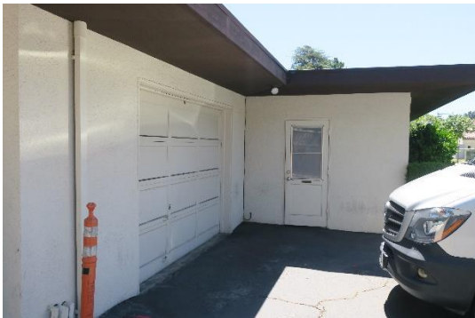
Figure 19: Roll-up wood paneled garage door and partially glazed wood door, view looking southeast.
