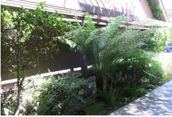
Figure 10: Lower portion of southeast-facing plane, clad in vertical wood siding, situated above a stone base planter.
