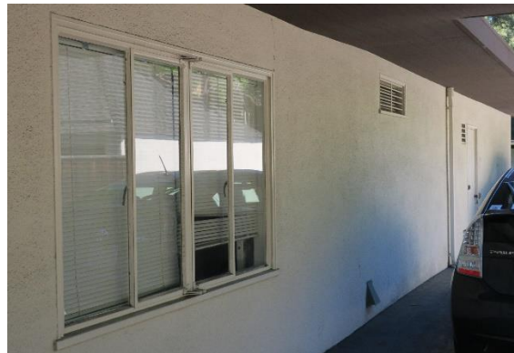
Figure 17. Two casement windows flanked by fixed lites, and wood door at image right, view looking south.
