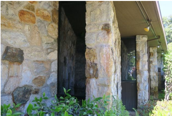
Figure 12: Sawtooth stone wall with fixed windows above wood siding, view looking northwest.
