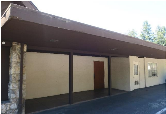
Figure 16: Recessed vestibule with cantilevered roof. Partially glazed door and paired casement windows at image right, view looking south.
