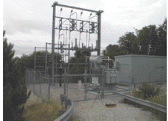
Figure 12: Typical Rail Corridor Paralleling Station
