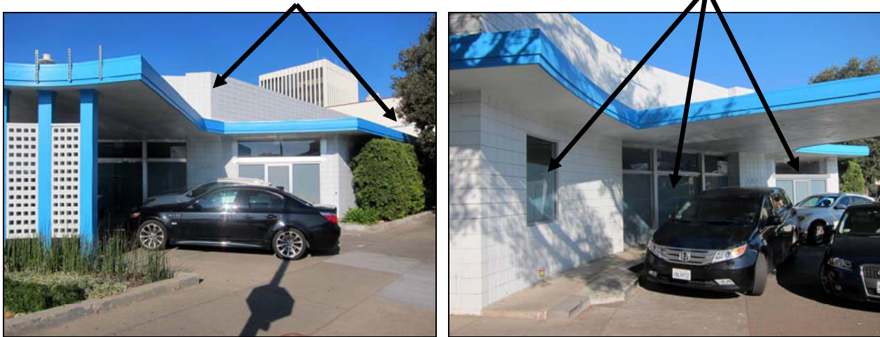
Figures 5 and 6. Left image shows a view down Forest Avenue with the addition shown between the arrows. Right image shows a detail of the angled entrance and replaced glazing (arrows).
