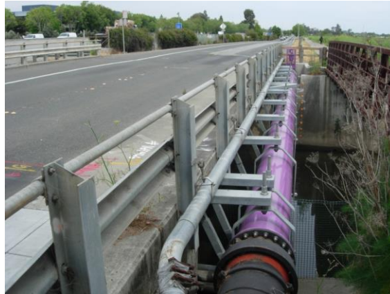
Figure 2-8: Example of a Recycled Water Pipeline Hung from Bridge
