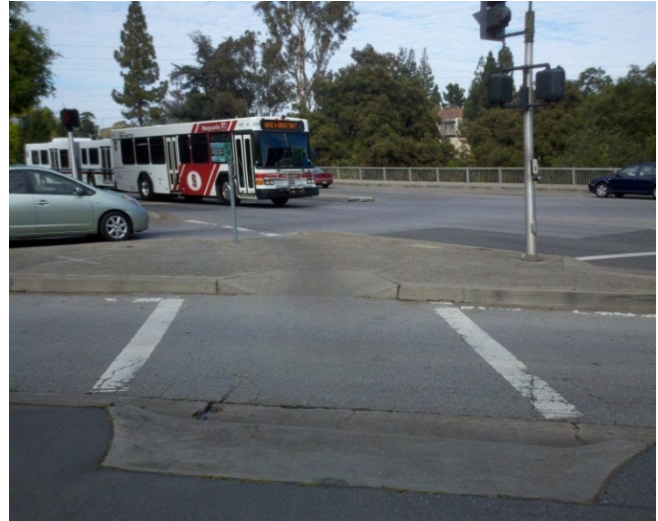
The series of non-conforming curb ramps and isolated islands across Palm Drive and the El Camino Real off ramps makes walking or biking to downtown or the transit center much less inviting.
