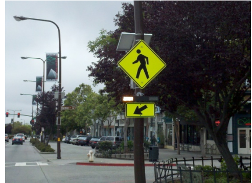
RRFBs can be solar powered and are an inexpensive alternative to full signalization. Note: City of Palo Alto standards call for a circular, as opposed to a rectangular, beacon signal head.
