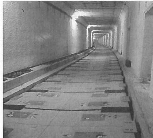
Figure 8 Photo of TTC double-tie system in subway - before installation of the rail fasteners and rail.
