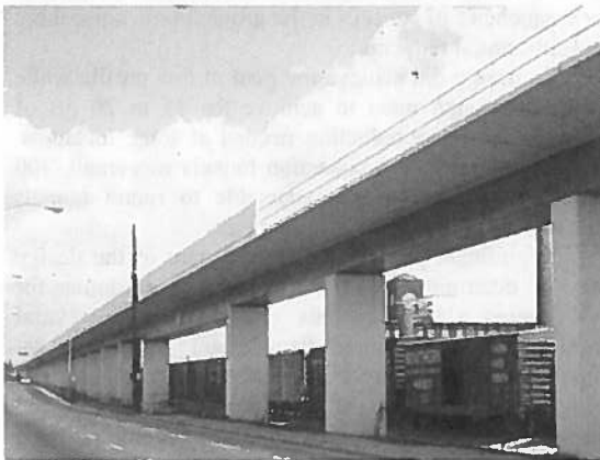
Figure 5 MARTA double track concrete deck with damped steel girder and sound barrier wall
