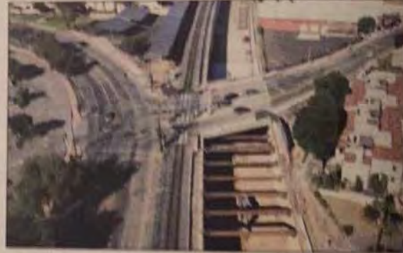
TRAIN IN A TRENCH — An aerial view of construction of a trench in San Gabriel in 2016. Photo by Brian O'Neil.
