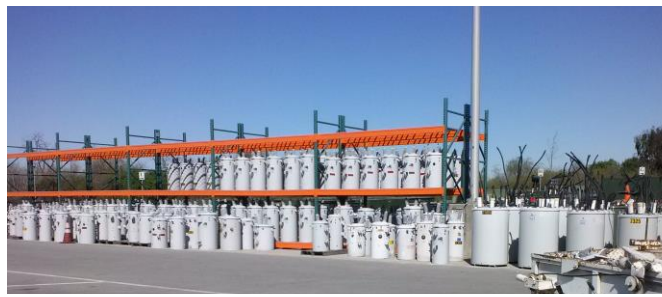
Exhibit 8: Transformers stored at the MSC
