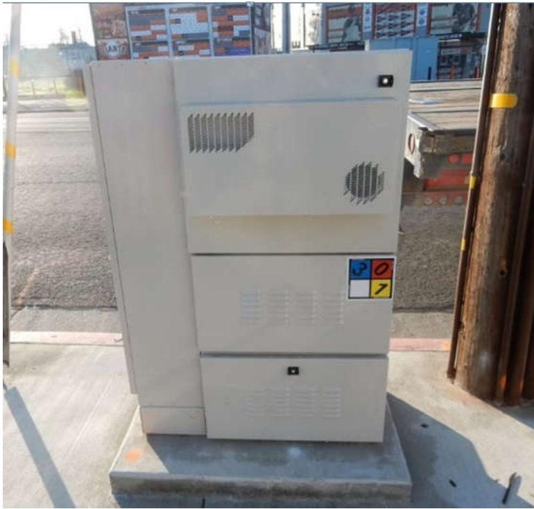
Ground-mounted emergency battery cabinet without wrap.
